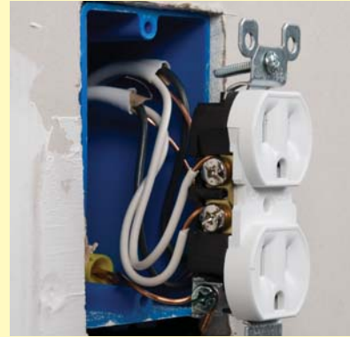
Screw terminal where a wire is connected to a receptacle may become loose as it is pushed back into the work box
