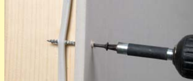
Accidentally piercing electrical cable behind drywalls with drill bit, nail, or screw
